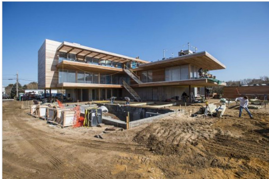
An oceanfront home being built by Fred G. Lappe General Contracting Inc. in Bridgehampton on March 20, 2014. (Credit: Gordon M. Grant)
